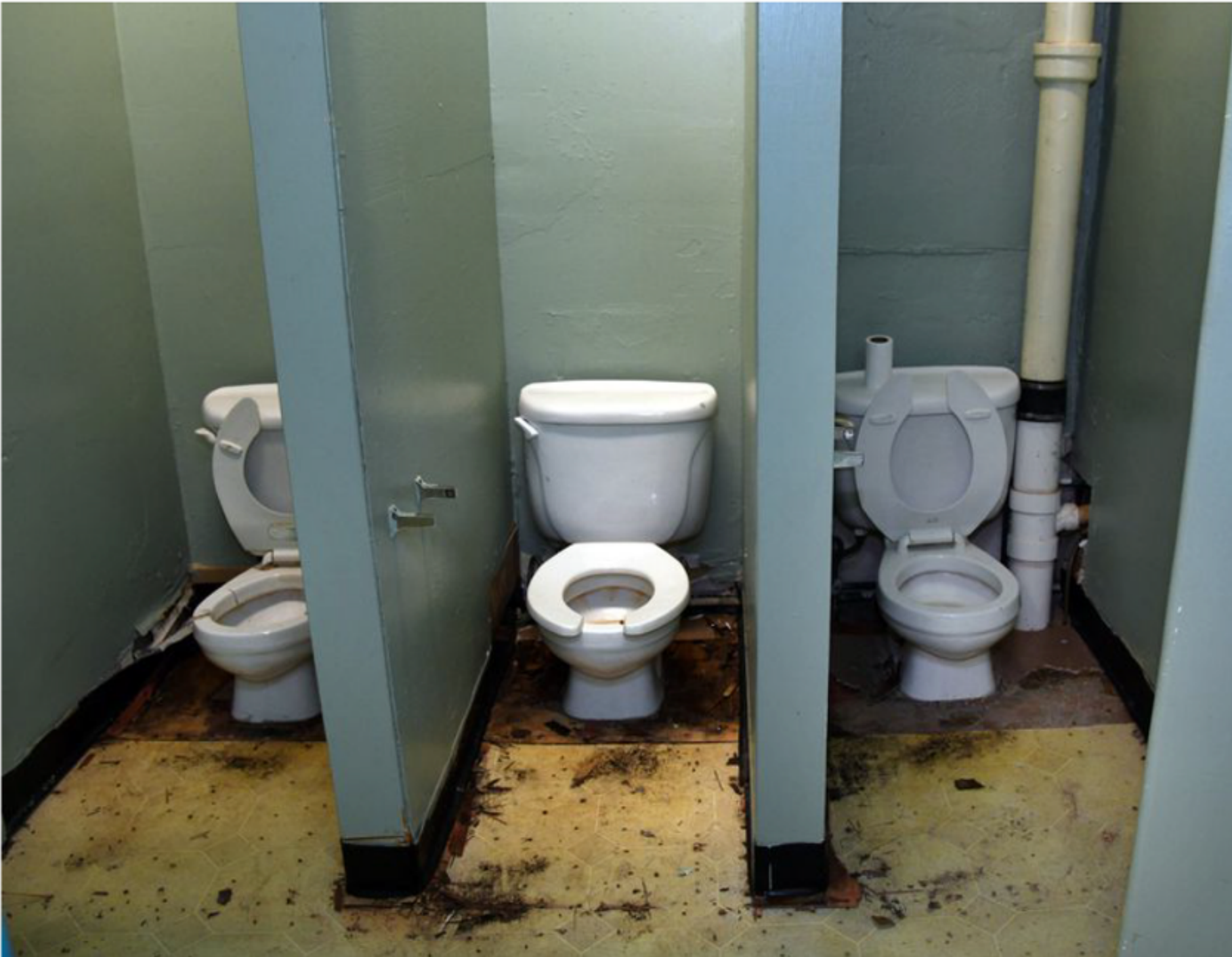
Aging infrastructure can result in sewage backups that can breed disease. (Barbara Haddock Taylor / Baltimore Sun)
